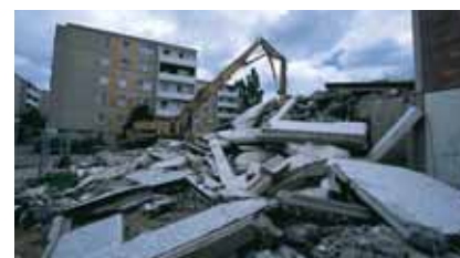
City of Frankfurt (Oder), Germany, has been experiencing population decline. The German federal government has been subsidizing demolition and removal of vacant buildings.
